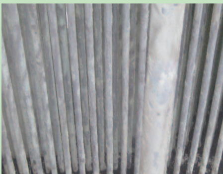
Above: Deposits on copper coil before Hybrid Cleaning.
