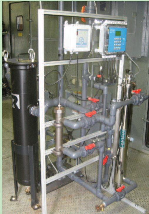
Above: eH 2 O Hybrid Condenser Cleaning water treatment system.
