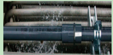
Above: Sprayers that clean condensing coil during operation.
